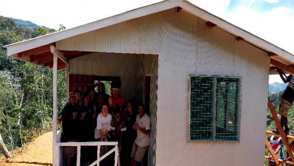
KALVARY HEALTH CLINIC - in the remote Central Highlands, staff accommodation block remains to be built.
